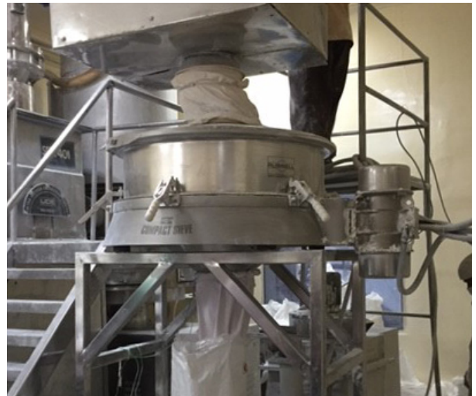
Figure 1. The Russell Compact Sieve® installed to screen pharmaceutical powders at Sri Krishna Pharma's Uppal factory
